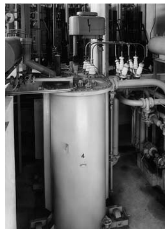
Switchgear in powerhouse building 2, transformer
