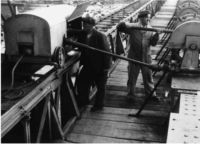
Weir, mobile engine driving the sluice gates
